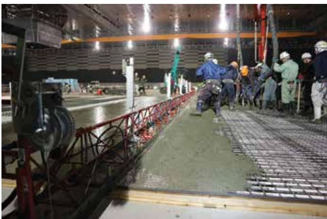
Shimizu Corporation workers placing concrete and screeding with end-to-end truss screeds. Note the lasers used to align the truss screeds
