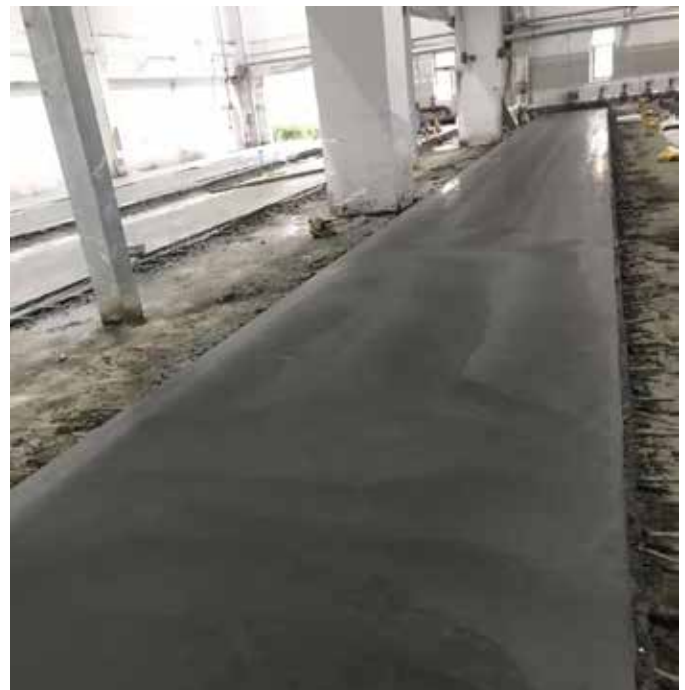
Finished floor at Harbin Medisan in Suihua, China, constructed by Shanghai WellRock Engineering Co.
