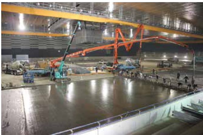
Pumping and striking off concrete for the speed-skating rink in Hachinohe, Japan, constructed by Shimizu Corporation. Note the laser projector overhead
